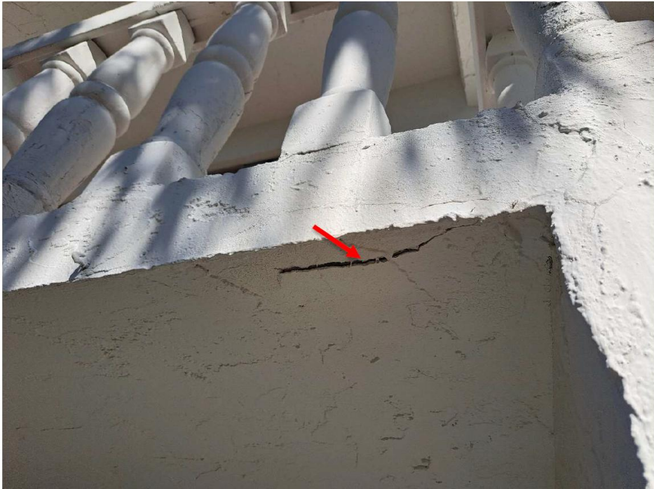
Photo 02 Ref: 2.1.1.1 – Slab Edge Spall, Unit #209’s Balcony (Typical)
