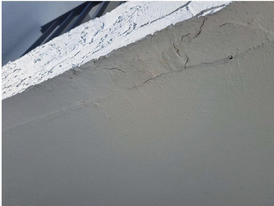
Photo 21 Ref: 2.1.3.1 – Spalled Stair Landing, East Tower
