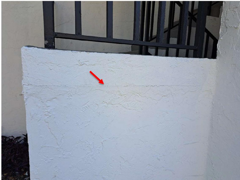
Photo 15 Ref: 2.1.3.1 – Crack Between Stair Landing Floor Slab & Wall, , West Tower
