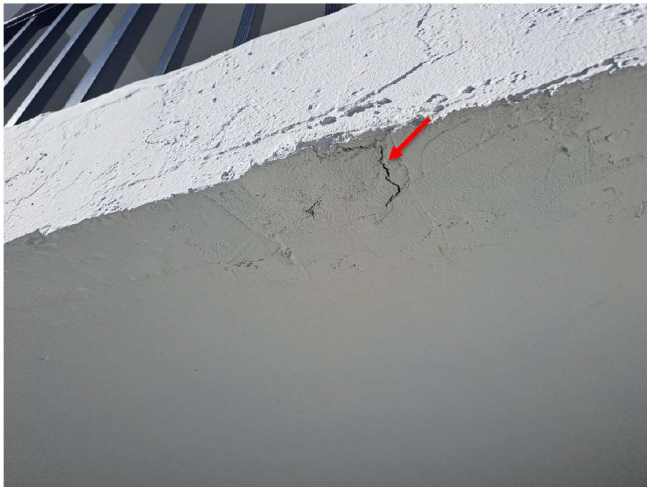
Photo 22 Ref: 2.1.3.1 – Spalled Stair Landing, East Tower
