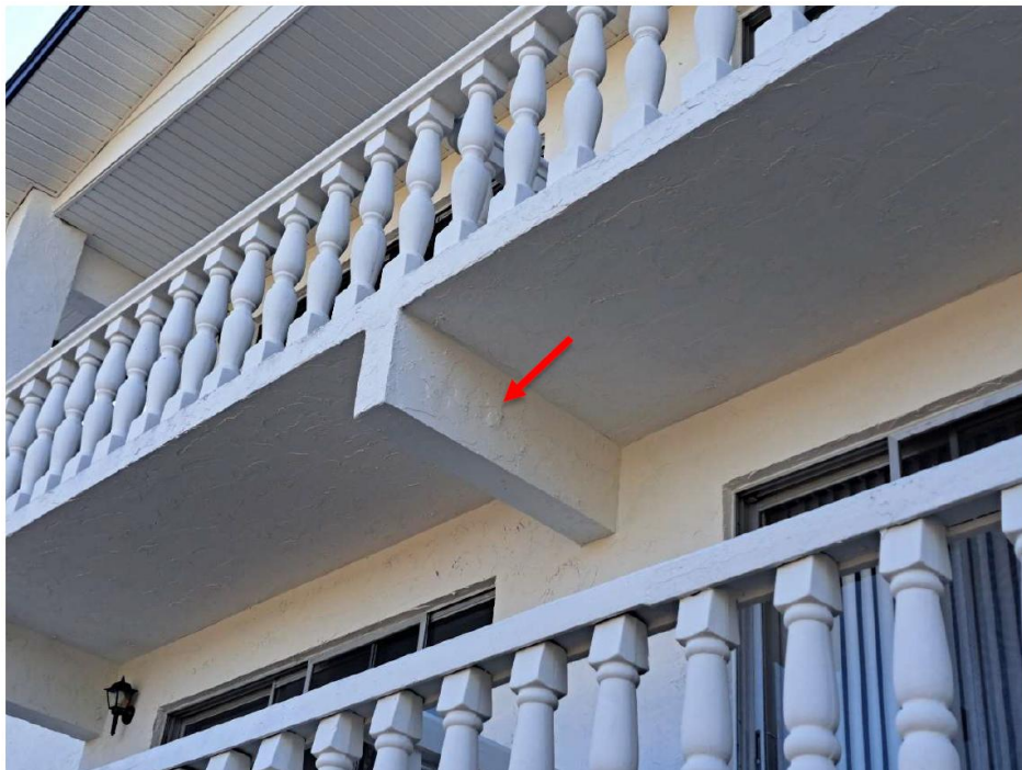
Photo 04 Ref: 2.1.1.1 – Support Beam Spall, Unit #304's Balcony (Typical)
