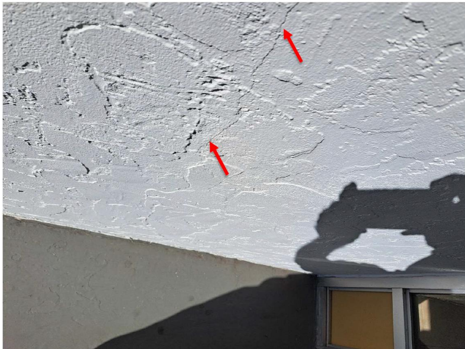
Photo 09 Ref: 2.1.2.1 – Crack In Entrance Wall, Pool Side
