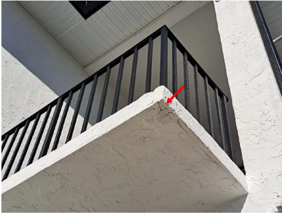
Photo 17 Ref: 2.1.3.1 – Spalled Stair Landing, East Tower
