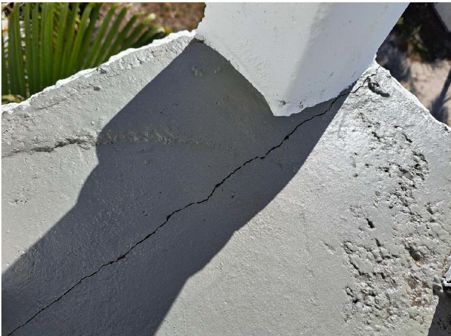
Photo 05 Ref: 2.1.1.1 – Cracked Slab, Unit #301's Balcony (Typical)
