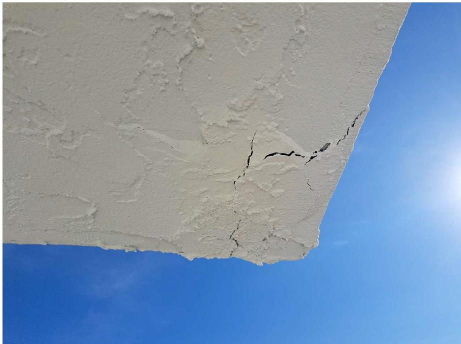
Photo 18 Ref: 2.1.3.1 – Spalled Stair Landing, East Tower
