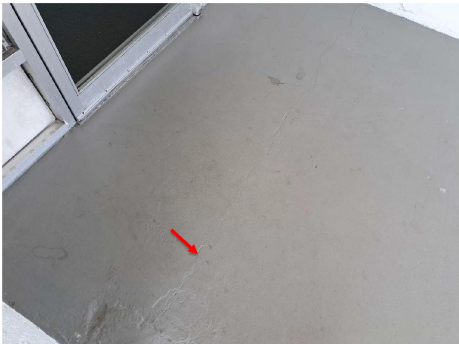
Photo 14 Ref: 2.1.3.1 – Crack In Stair Landing Floor Slab, , East Tower (Typical)
