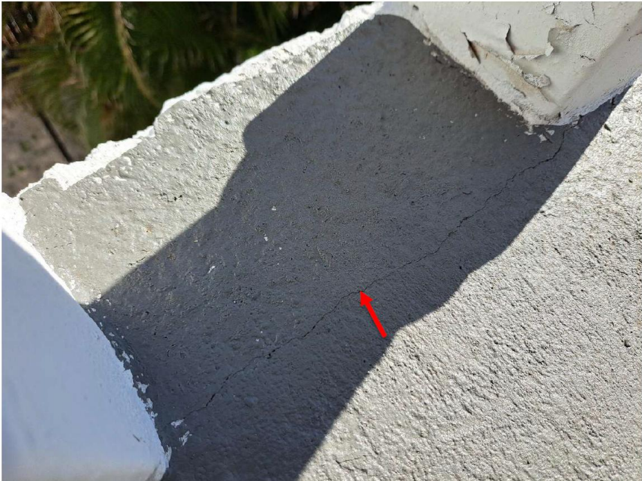
Photo 06 Ref: 2.1.1.1 – Cracked Slab, Unit #321's Balcony (Typical)
