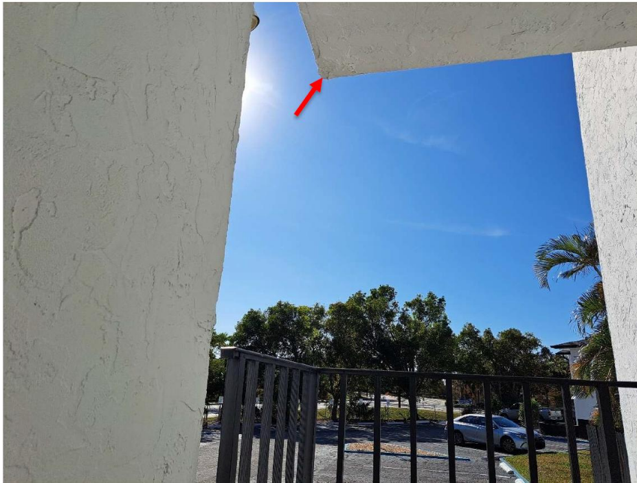
Photo 19 Ref: 2.1.3.1 – Spalled Stair Landing, East Tower
