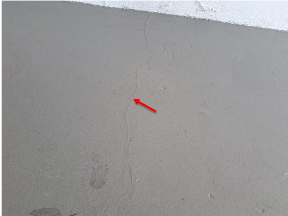
Photo 13 Ref: 2.1.3.1 – Crack In Stair Landing Floor Slab, , East Tower (Typical)
