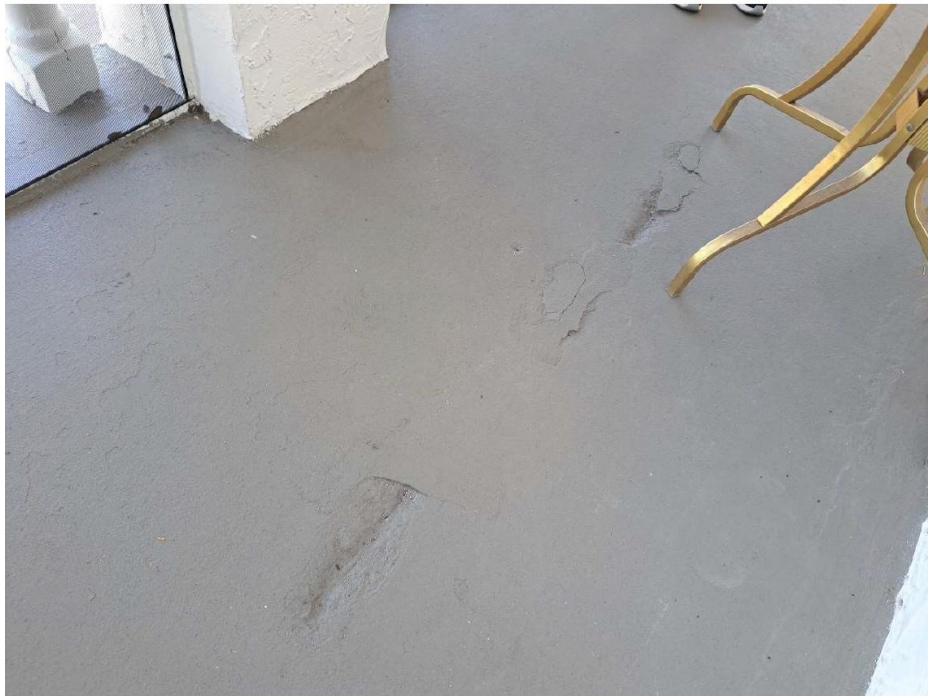
Photo 07 Ref: 2.1.1.1 – Spalled Slab w/ Exposed Rebar, Common Room Balcony
