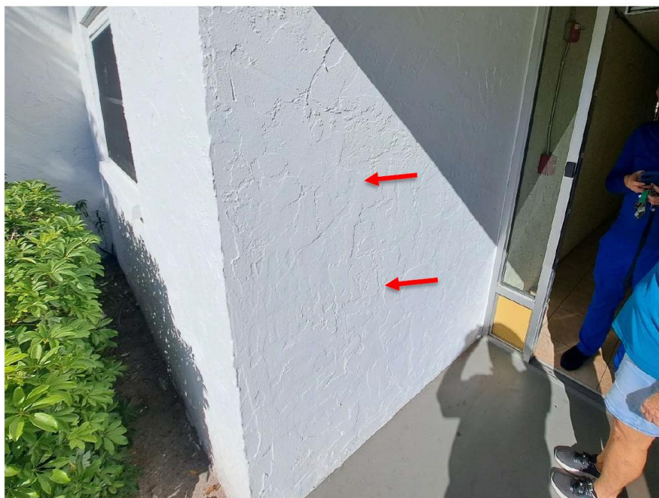
Photo 10 Ref: 2.1.2.1 – Crack In Entrance Wall, Pool Side
