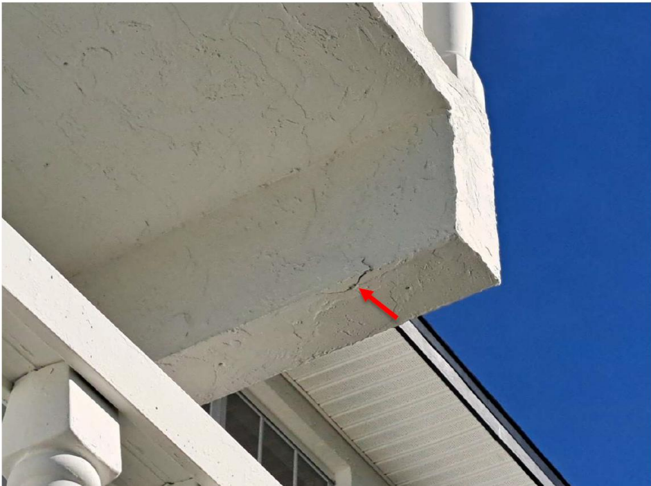
Photo 01 Ref: 2.1.1.1 – Support Beam Spall, Unit #313’s Balcony (Typical)
