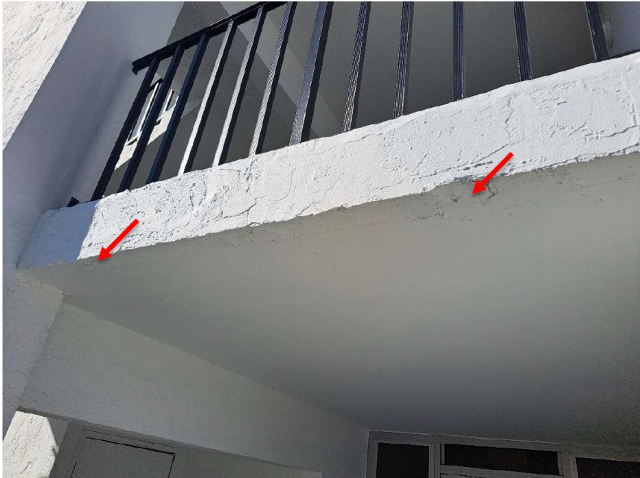
Photo 23 Ref: 2.1.3.1 – Spalled Stair Landing, East Tower
