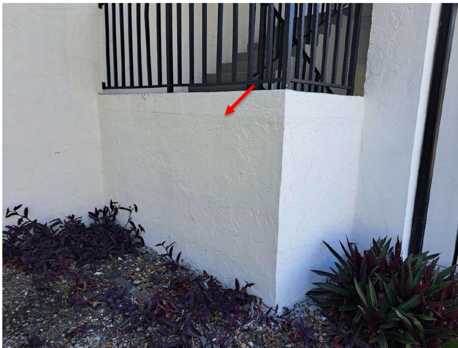
Photo 16 Ref: 2.1.3.1 – Crack Between Stair Landing Floor Slab & Wall, , West Tower
