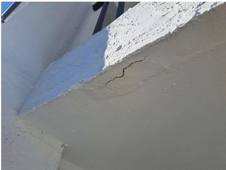
Photo 20 Ref: 2.1.3.1 – Spalled Stair Landing, East Tower
