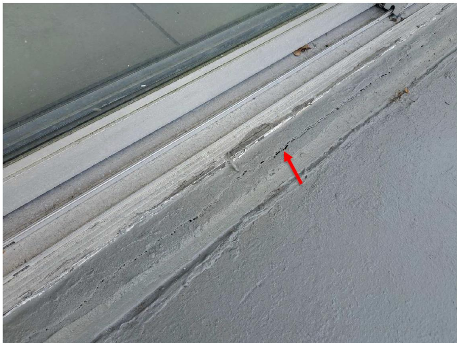
Photo 08 Ref: 2.1.1.1 – Spalled Door Sill, Unit #320's Balcony (Typical)
