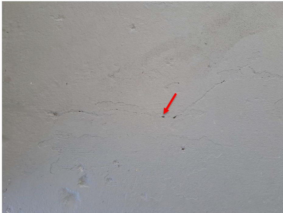
Photo 12 Ref: 2.1.3.1 – Crack In Stair Landing Floor Slab, , East Tower (Typical)
