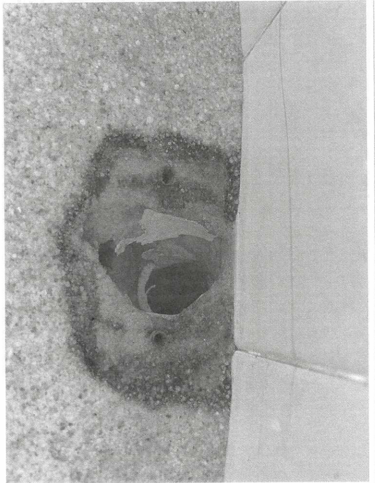
Leaks found at four gutter ports
