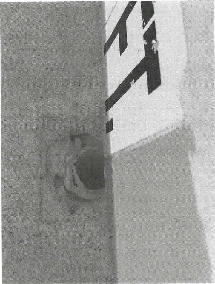
Leaks found at four gutter ports
