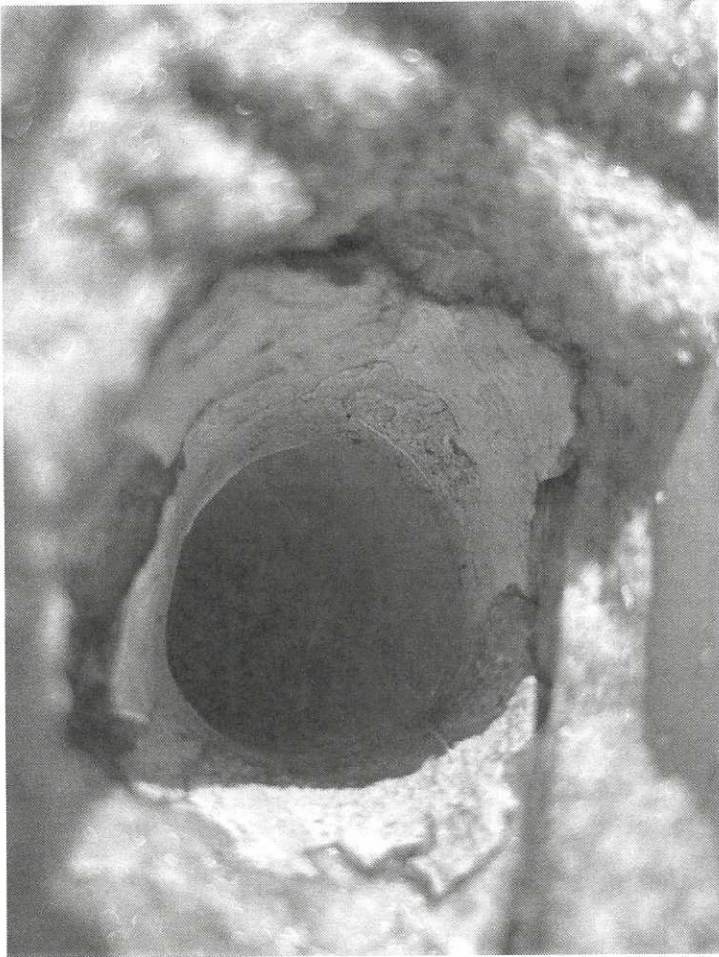
Leaks found at four gutter ports
