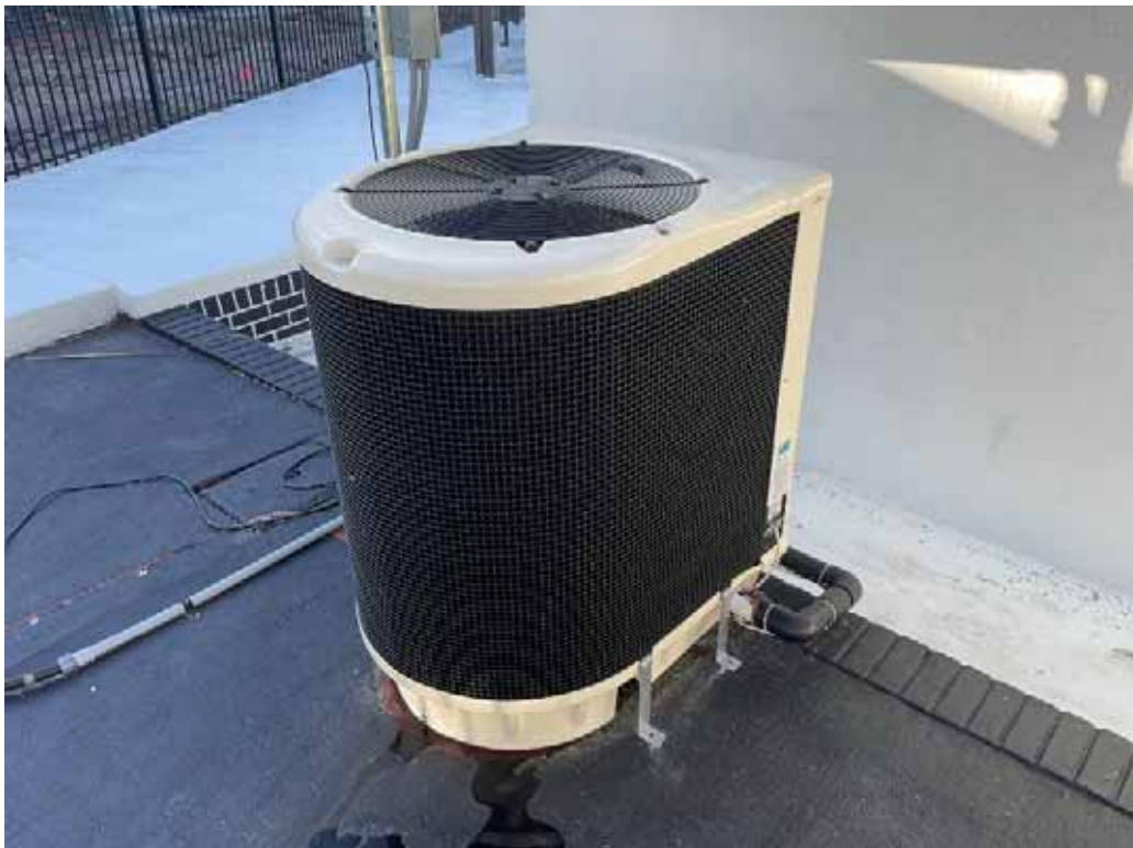
Pool Equipment, Heater
