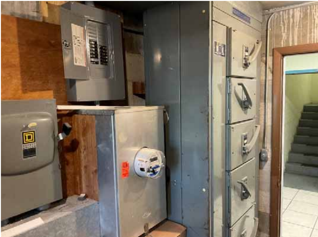
Bldg A Main Electrical Switchgear
