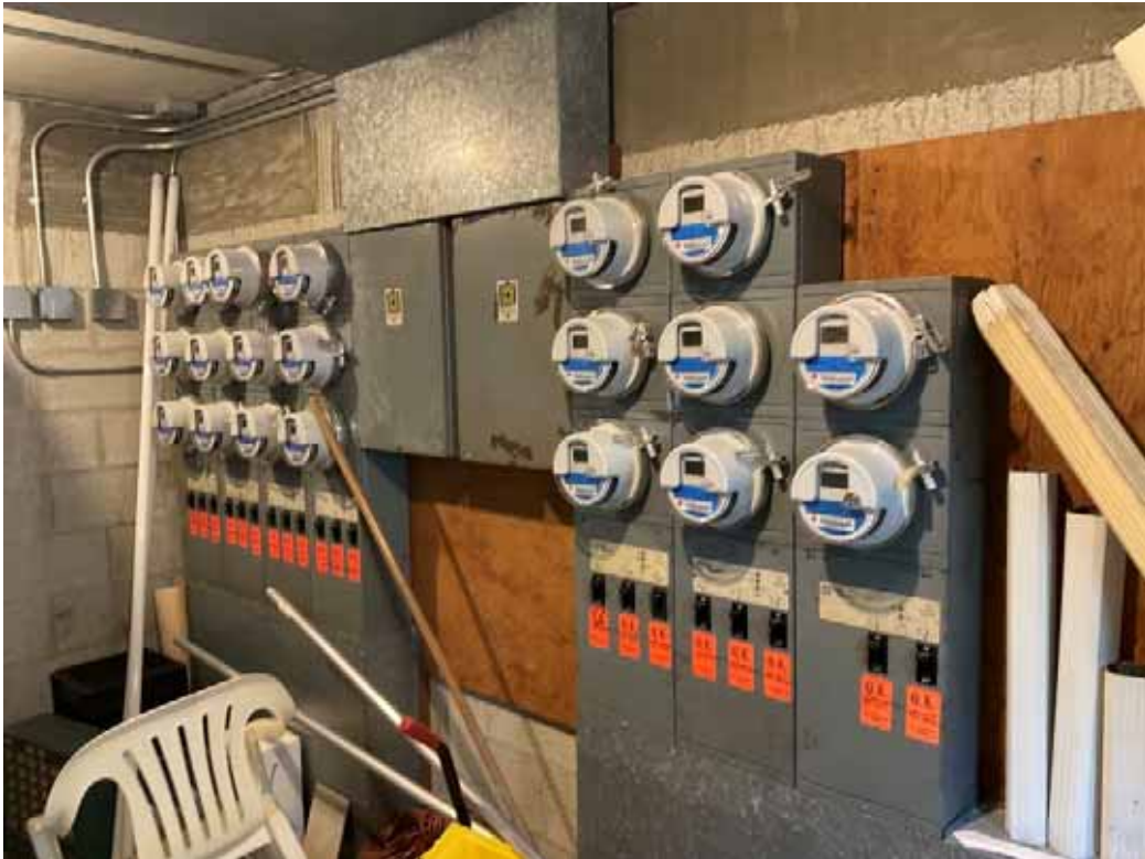
Bldg A Electrical Meters
