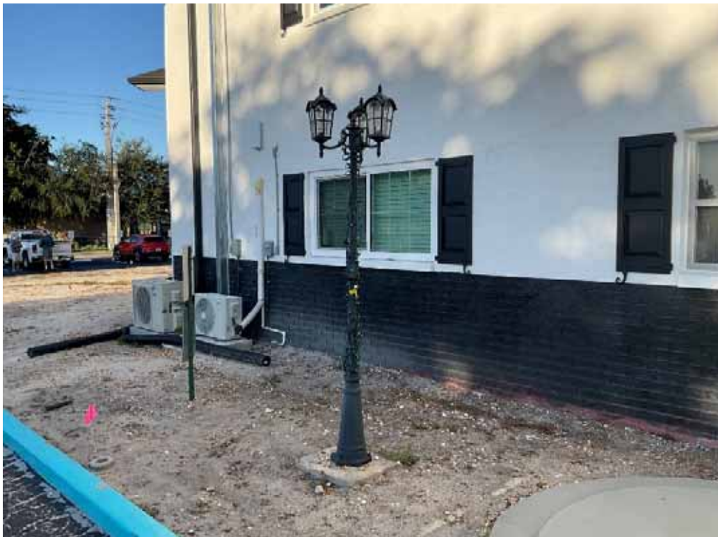
Light Pole & Fixtures - Parking Lot
