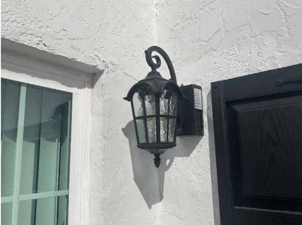
Bldg A Common Area Lighting
