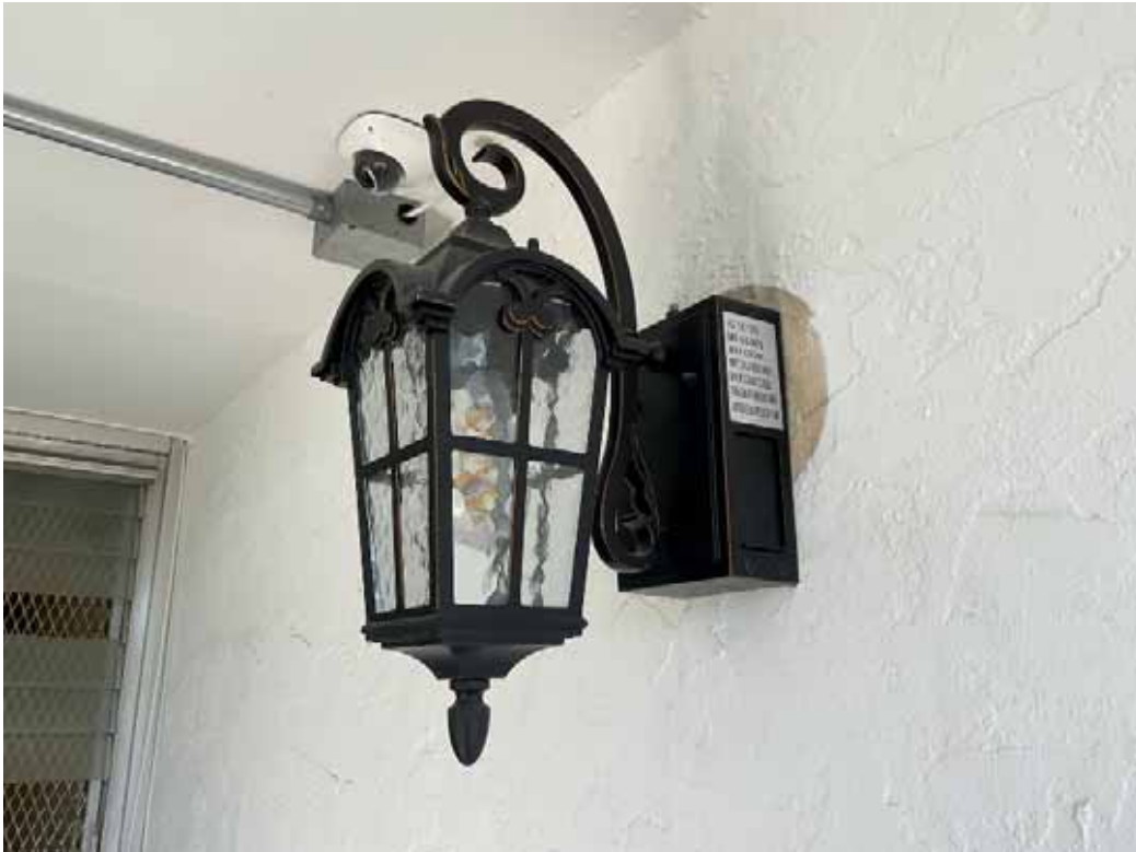
Bldg B Common Area Lighting
