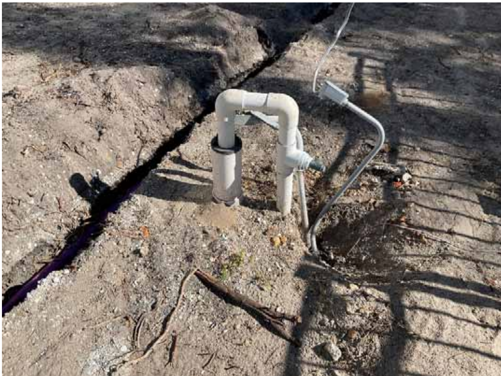
Irrigation Well Pump Station
