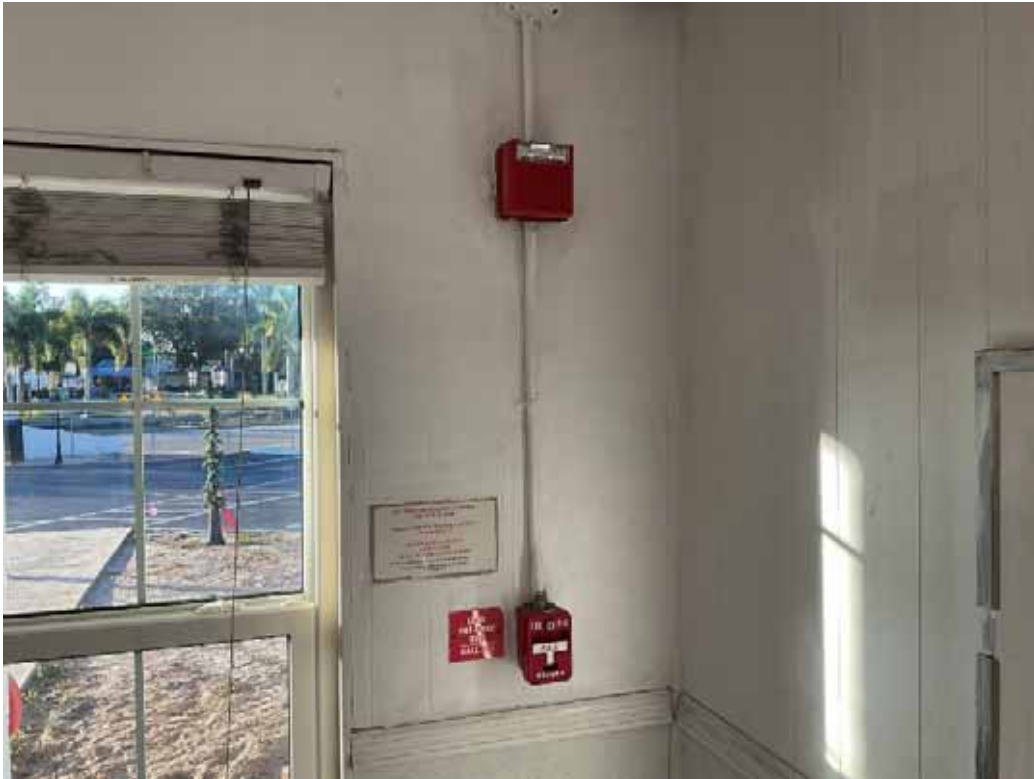
Bldg A Fire Alarm System Equipment
