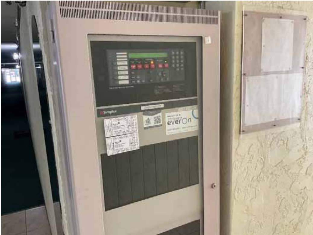
Bldg B Fire Alarm Panel
