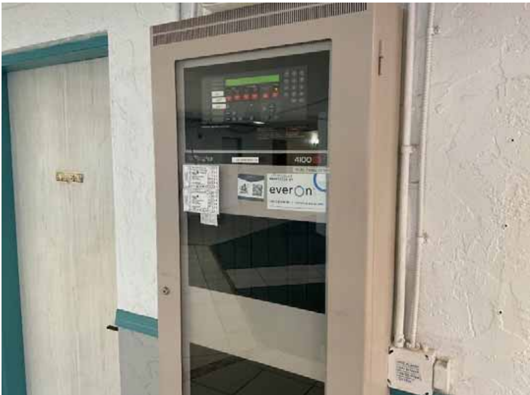
Bldg A Fire Alarm Panel
