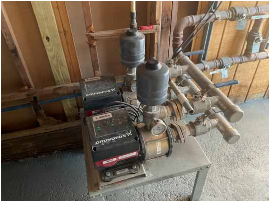
Domestic Water Booster Pump System - Condo Bldgs
