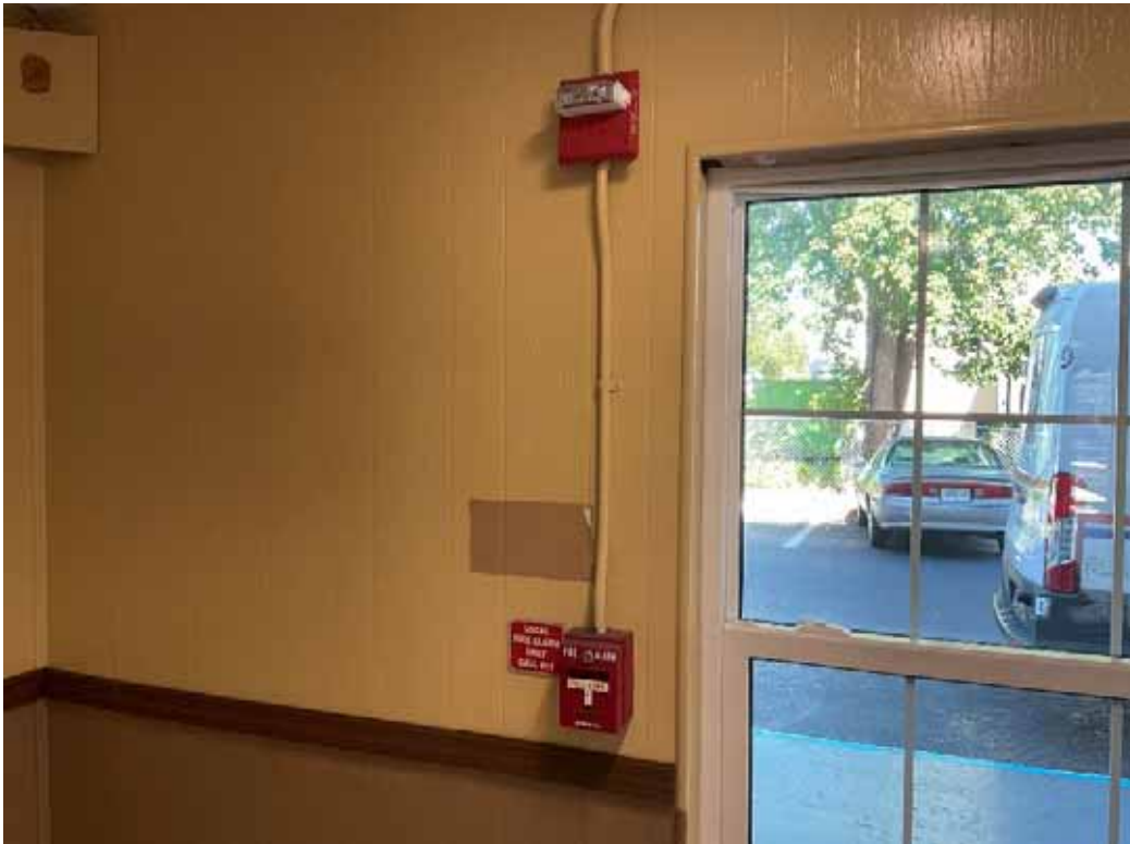
Bldg B Fire Alarm System Equipment
