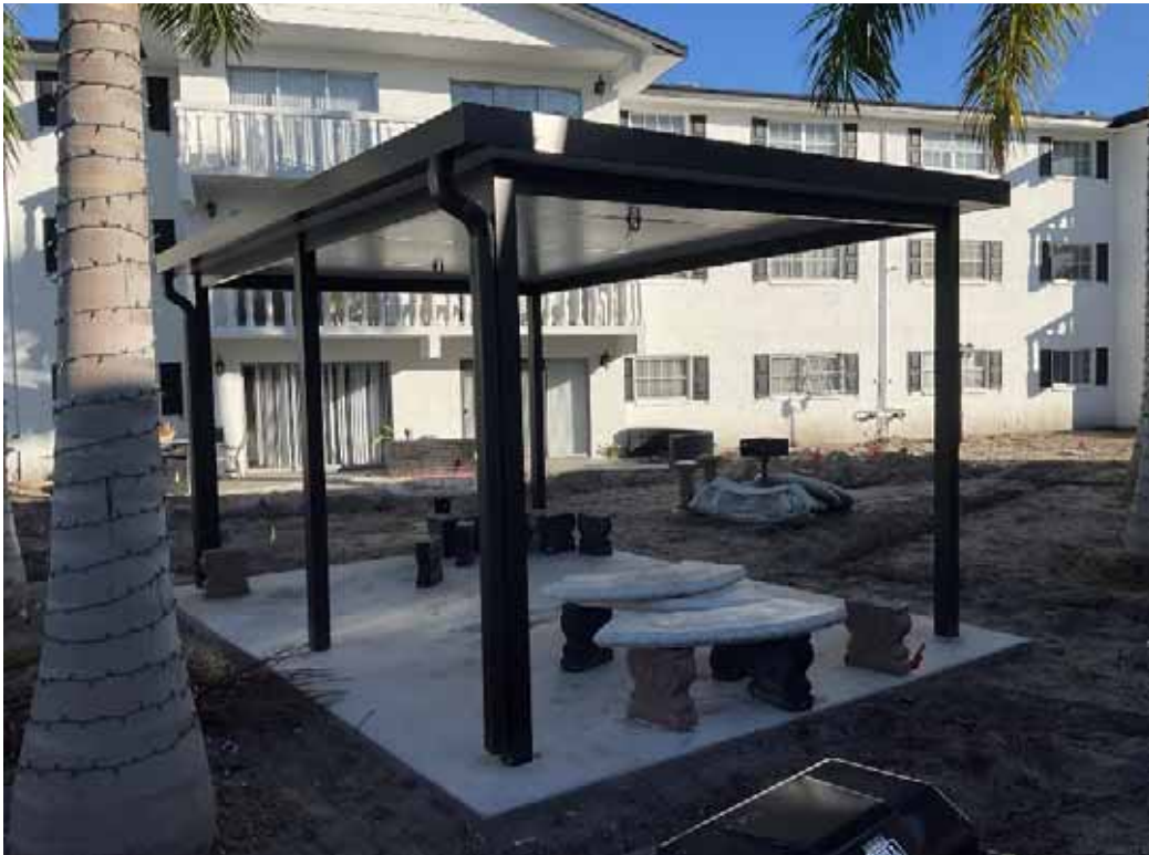
BBQ Area Shade Shelter
