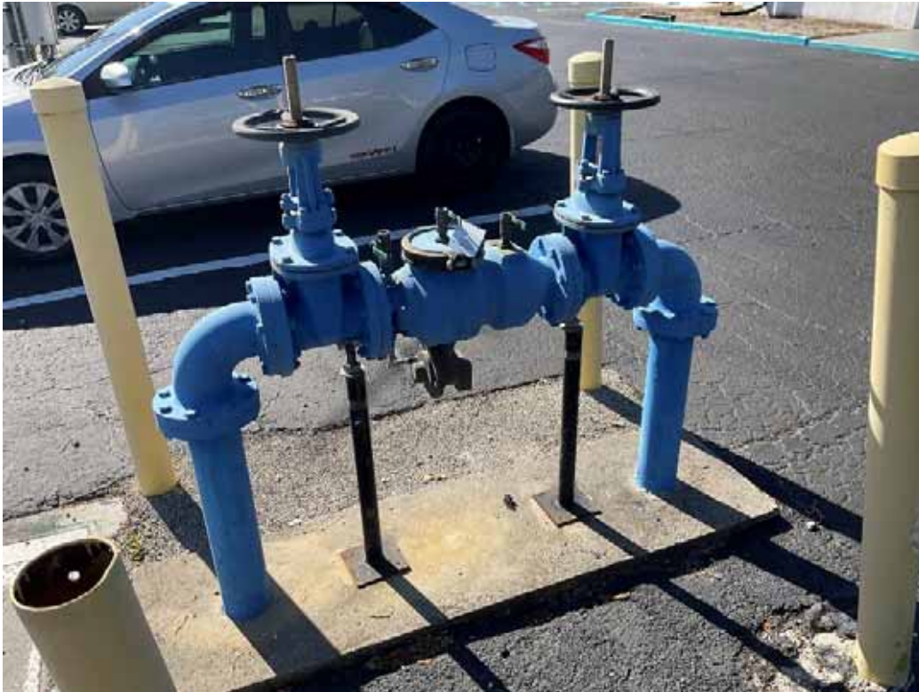
Backflow Preventer - Domestic Water
