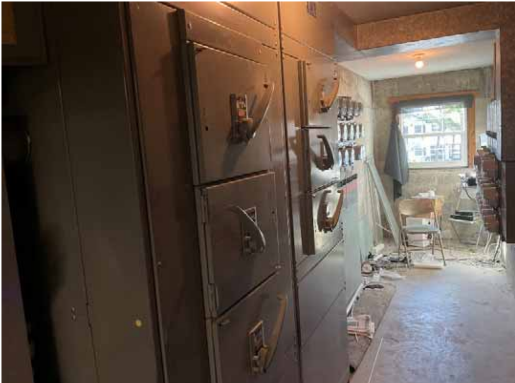
Bldg B Main Electrical Switchgear
